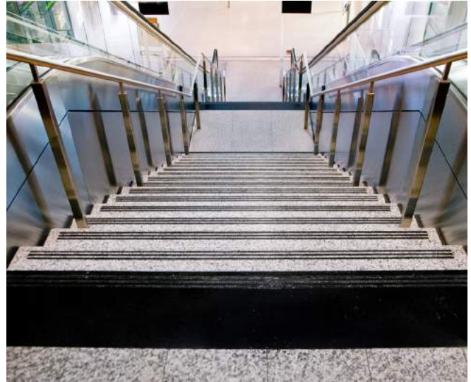
An example showing poor use of stair nosings. The light-coloured treads with black strips on the nosing create a marking pattern that is not perceived well by people with vision loss.
