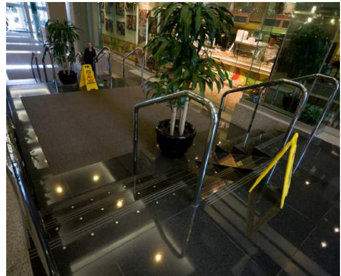
An example of poor stair design – black stairs with no colour contrast on the nosing.
