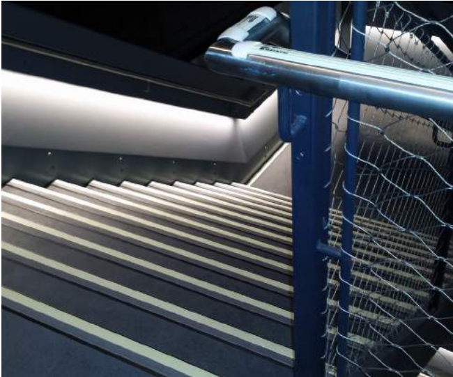
A good example of universal design for stairs. Nosings incorporate good colour contrast.
